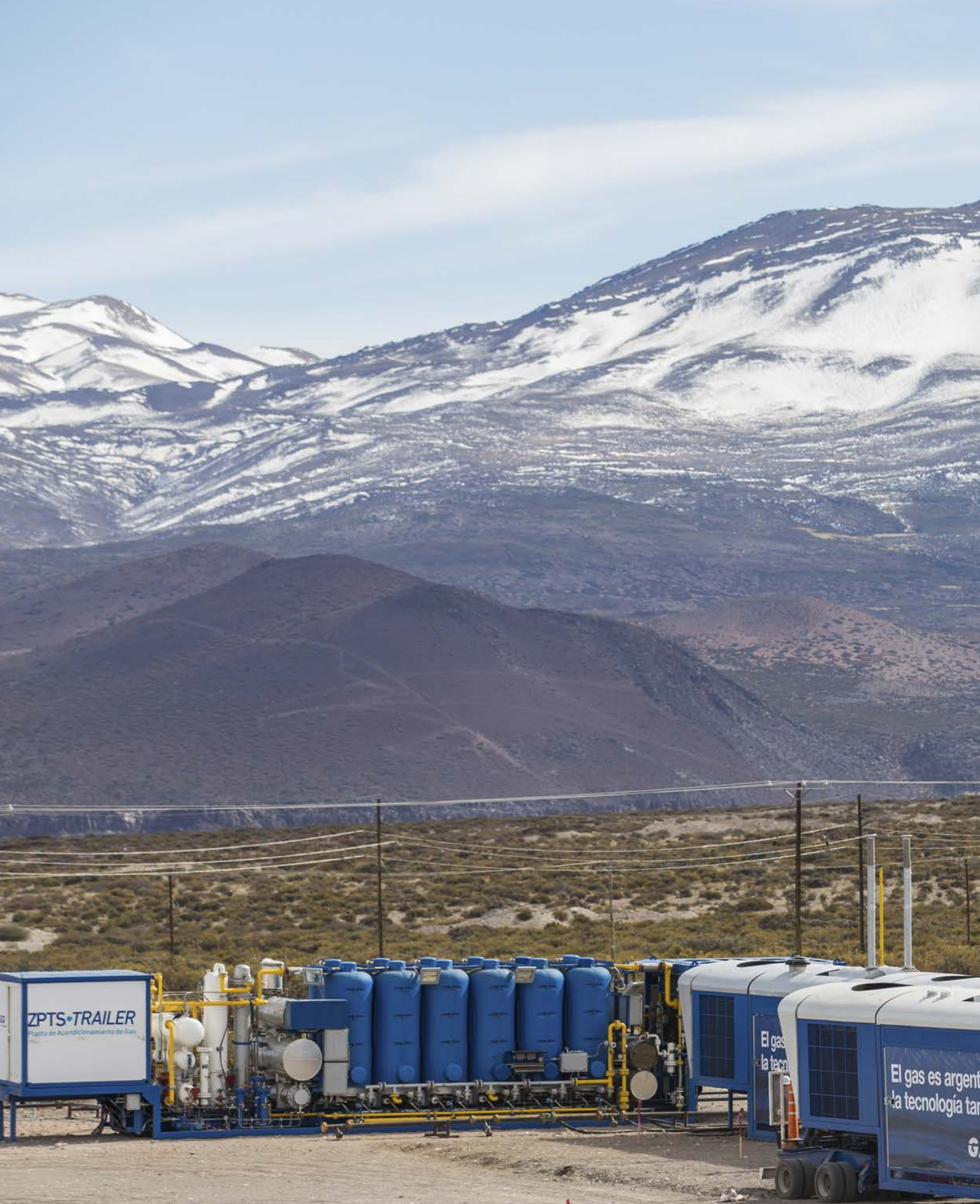
Figure 2. Two Cryobox® trailers at a remote well site in the Mendoza province coupled to a third trailer on which gas pre-treating equipment is installed to prepare the gas for liquefaction (courtesy of Galileo technologies).
